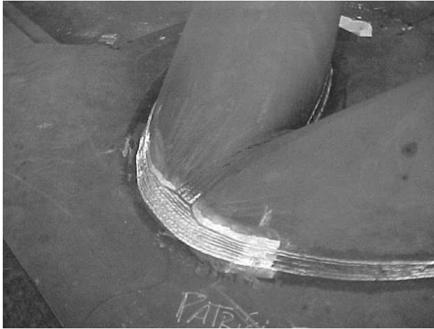
Figure 7 : Grinded node welds.
