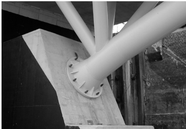
Figure 3 : Arch spring clamped by prestressing bars.
