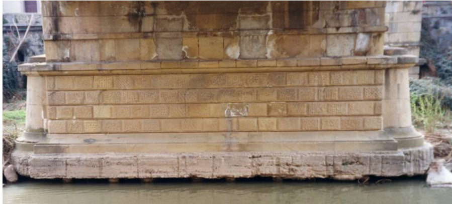
Figure 5 : Picture of the pier where piles are partly visible between the pile-cap and the water level.
