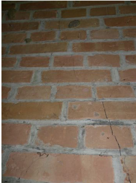
Fig. 7. Detail of a crack in barrel arch.
