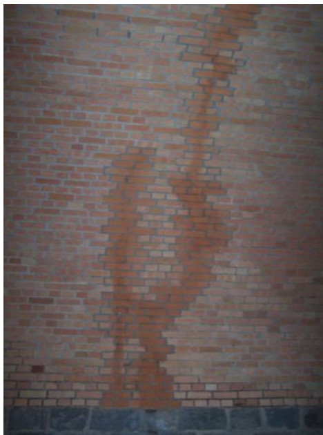
Fig. 8. Cracks after repair.
