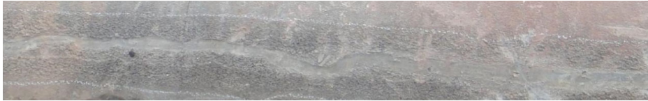
Fig. 8. The apparent water/air passage on segment 2-26.
