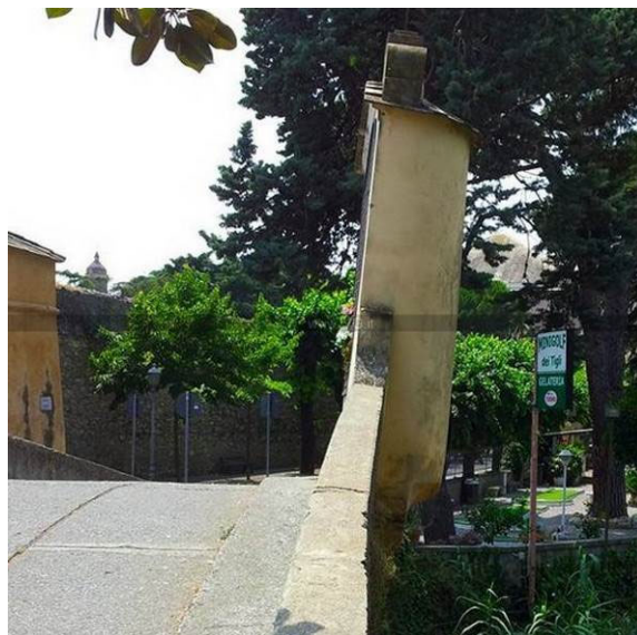
Fig. 4. Few hours before the collapse.
