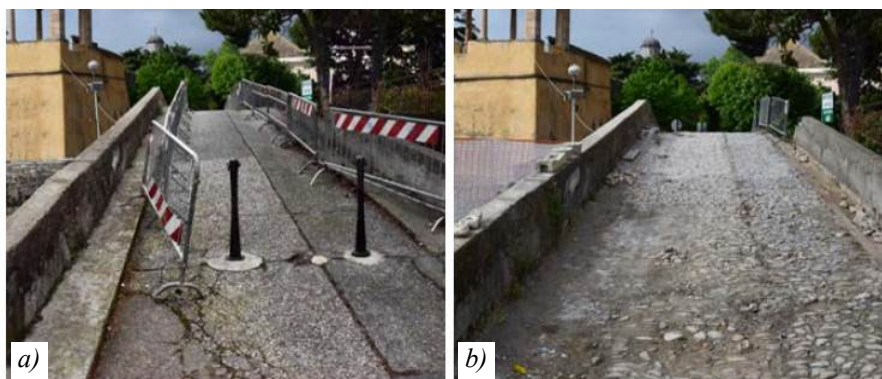
Fig. 3. a) Concrete pavement (1960 approx.). b) Original cobblestone on the right (after removal of the concrete layer). The southern side is on the left. On the right the „hole” in the spandrel due to the collapse of the aedicule.
