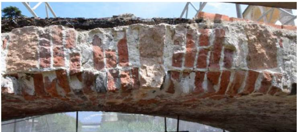
Fig. 6. Frontal view of the cracked surface.
