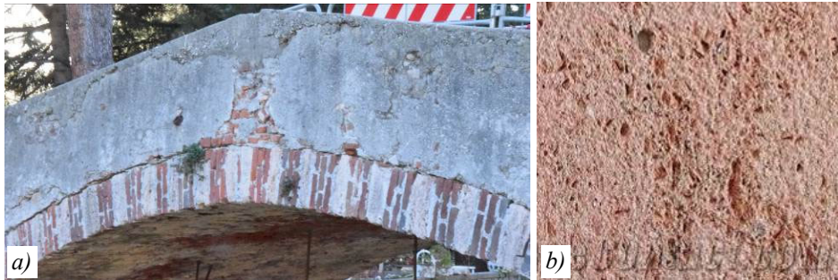
Fig. 7. a) Spandrel on the south side: bad conditions and sliding (?) at the arch-spandrel interface; b) texture of the Finale Stone (rose type).
