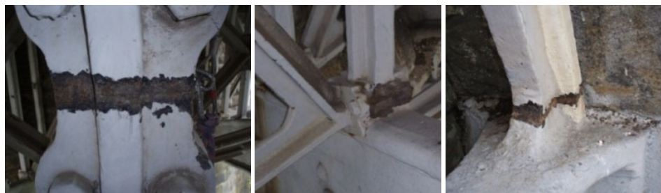
Fig. 10. Crack in vertical posts, ribs connections and bracing to ribs connection.
