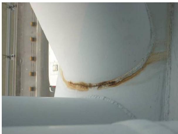
Fig. 1. Fatigue distress of Yajisha Bridge.
