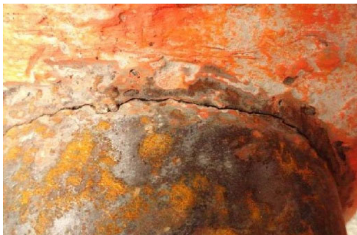
Fig. 2. Fatigue distress of Shitanxi Bridge.
